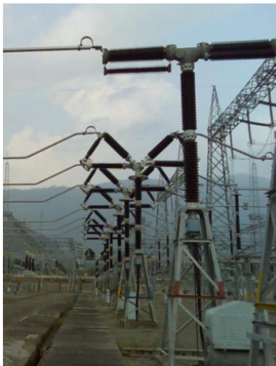
400 kV SF 6 live tank circuit breakers
