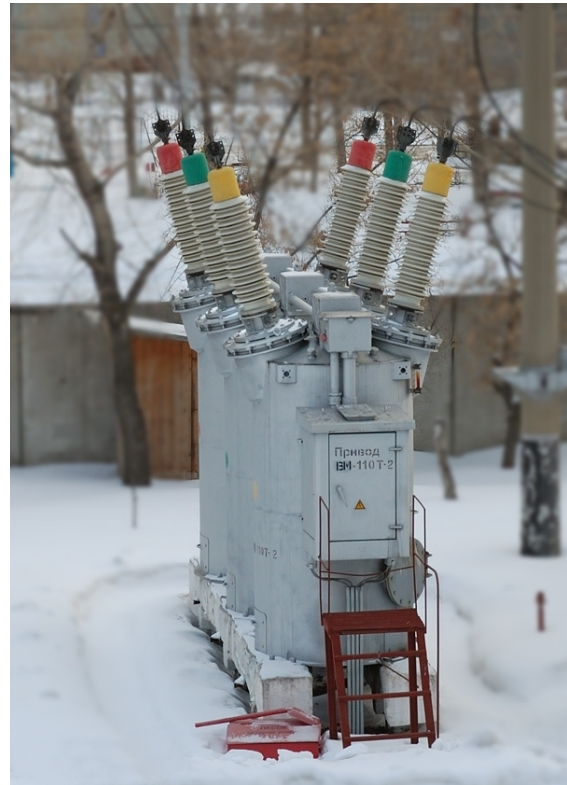
Three single phase Russian 110 kV oil circuit breakers
