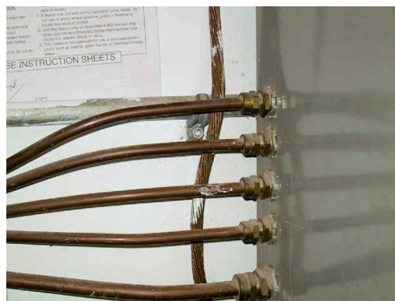
Mineral insulated cables at a panel board
