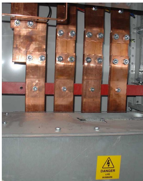
Copper is widely used for power distribution bus bars because of its high conductivity
