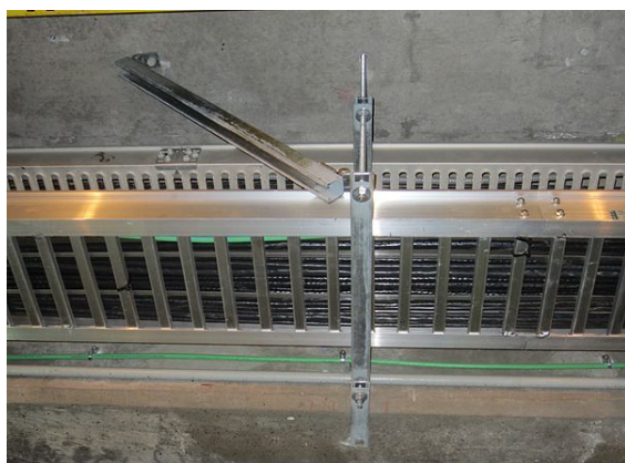
Seismic bracing of a cable tray trapeze support. The diagonal strut and horizontal tie restrains motion longitudinally and laterally.
