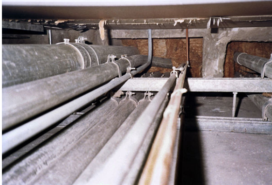
This illustration shows electrical conduit risers, looking up inside a fire-resistance rated shaft, as seen entering bottom of a firestop. The firestop is made of firestop mortar on top and mineral wool on the bottom. Raceways are used to protect cables from damage.
