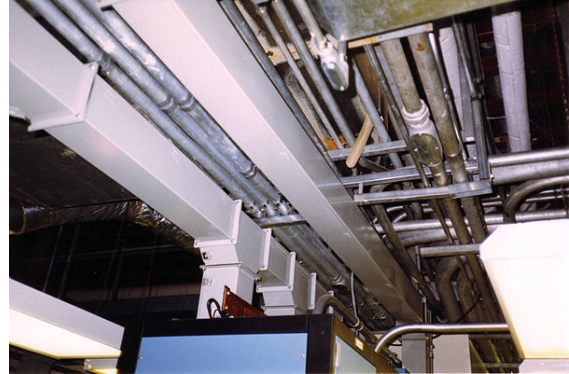
Electrical conduit and bus duct in a building at Texaco Nanticoke refinery in Nanticoke, Ontario, 1980s.
