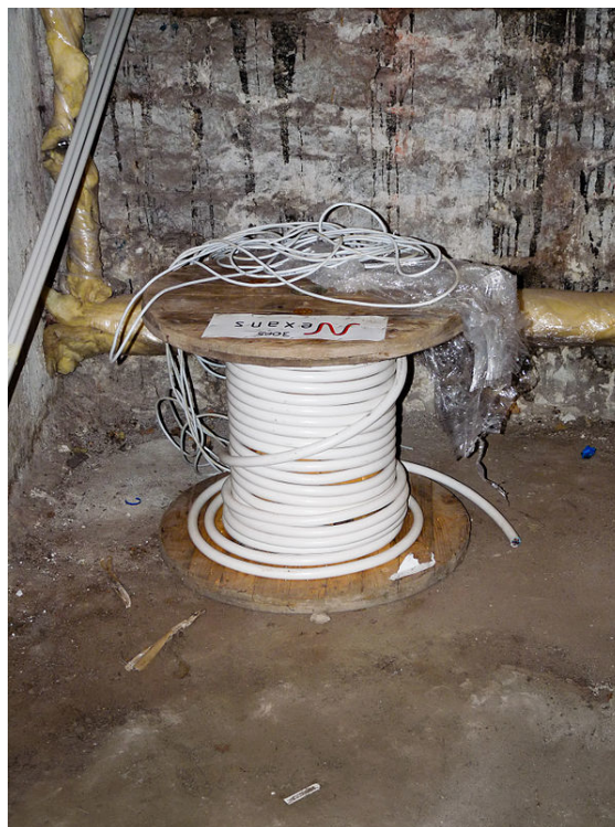
Power cable 5G16 (5 wires, green-yellow ground wire, 16mm 2 ).
