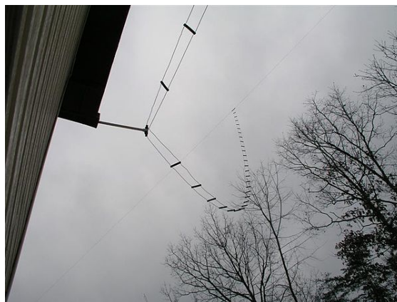
600 ohm “Ladder line” on the outside of a building.
