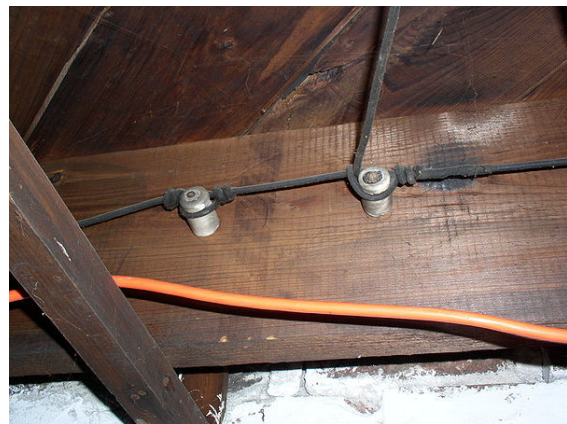
Knob-and-tube wiring (the lower pipe is an unrelated copper water line)
