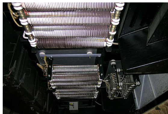
High-power wire wound resistors used for dynamic braking on an electric railway car. Such resistors may dissipate many kilowatts for an extended length of time.
